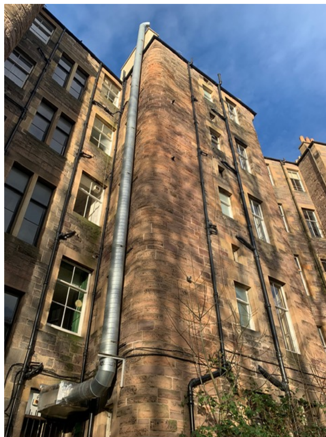
NEIGHBOURS AT No.171 EXISTING GALVANIZED EXTRACT DUCT
